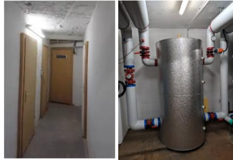
Limited space in the boiler room
