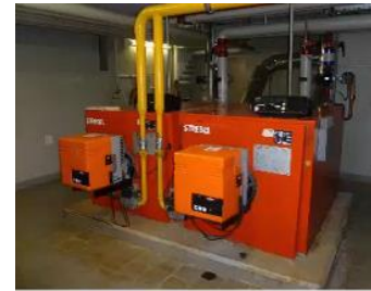
Keep existing equipment
