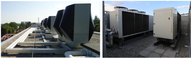
HP weight in the roof
